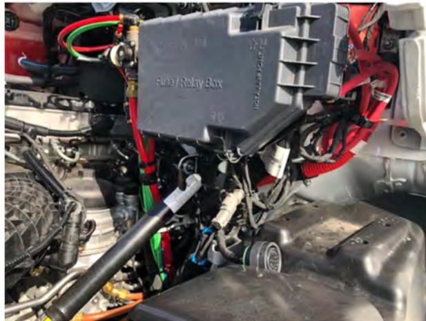
Fig 229, Power Distribution Module (PDMe) in Engine Compartment
